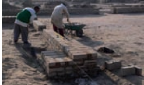
Local builder Mohammed Mahmoud Hussein at work, recreating the line of the front wall of the animal building.
